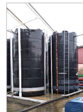
SMM's rainwater tanks
