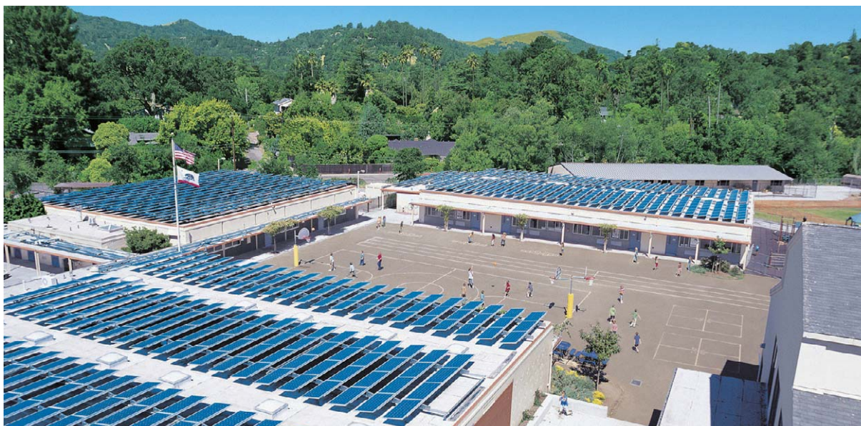
Photovoltaic power generation systems installed at an elementary school in California
