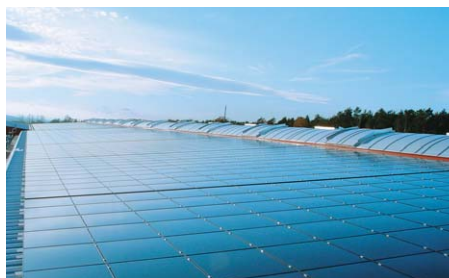
Thin-film solar cells installed at a company in Germany
