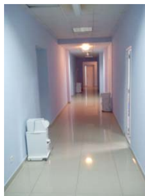
Photo: Plasmacluster ion device experimental installation in the hospital corridor
